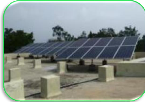
40 kW Solar Power Unit at Nava Bharat Schools, Paloncha
