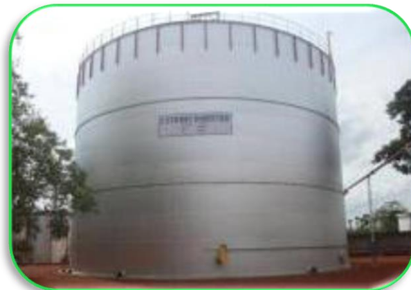
CSTR Bio-Digester to recover biogas & to use as fuel to distillery boiler
