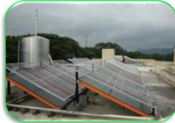
Solar water heaters at Dhenkanal & Paloncha
