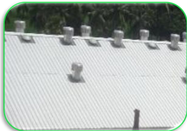
Turbo Ventilators at Dhenkanal & Samalkot
