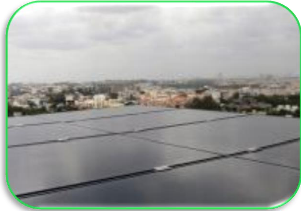
High Efficiency roof top solar power plant at Silicon House
